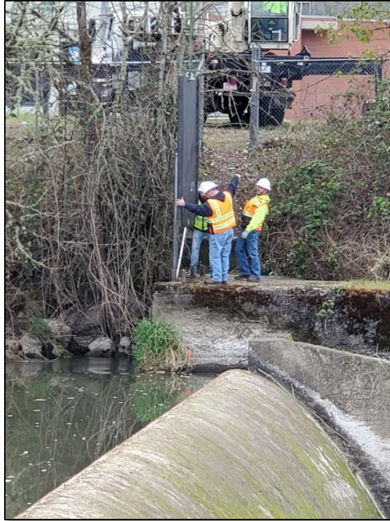
City of Monroe and City of Harrisburg's Public Works teams working together to install new sluzice gate. City of Monroe image.
