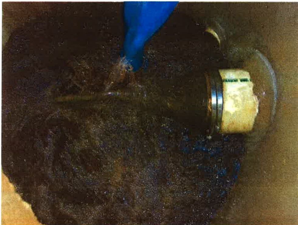
Exterior Inlet, and Overflow with Duckbill Valve
